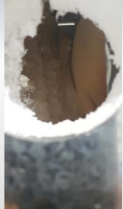
Cavity inside wall showing where EPS foam melted but GigaFoam stayed intact
